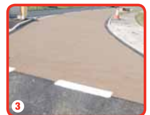
3 After resin mix has set, excess aggregate is brushed off before tape is removed leaving clean, straight finish
