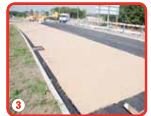
3 Surface is complete and can be ready for traffic in under an hour
