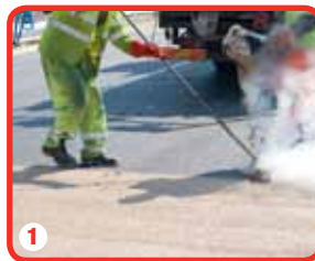
1 Area is cleared of debris before product is applied with a screed box
